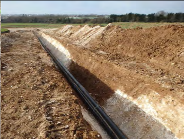
G76 exposed in cable trench looking south-west
