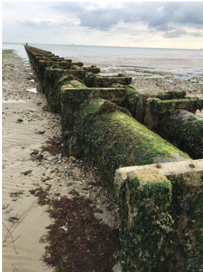
Southern Water outfall
